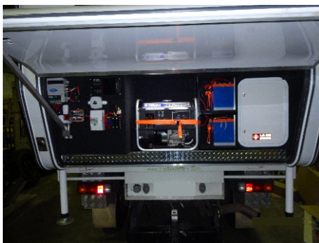
Storage / generator, battery management
